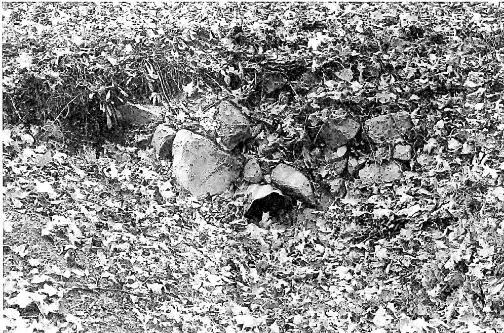
Picture #5 - Multiple driveway culverts are undersized, over vegetated, and full of debris
