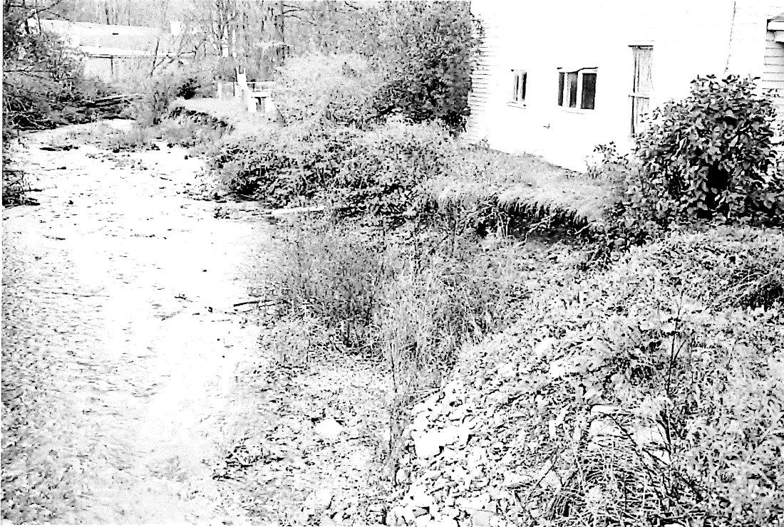
Picture #1 - Eroded banks along White Creek; facing east from bridge
