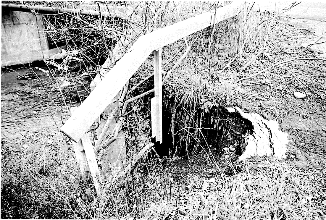
Picture #2 - Eroded banks, compromising bridge infrastructure; facing west
