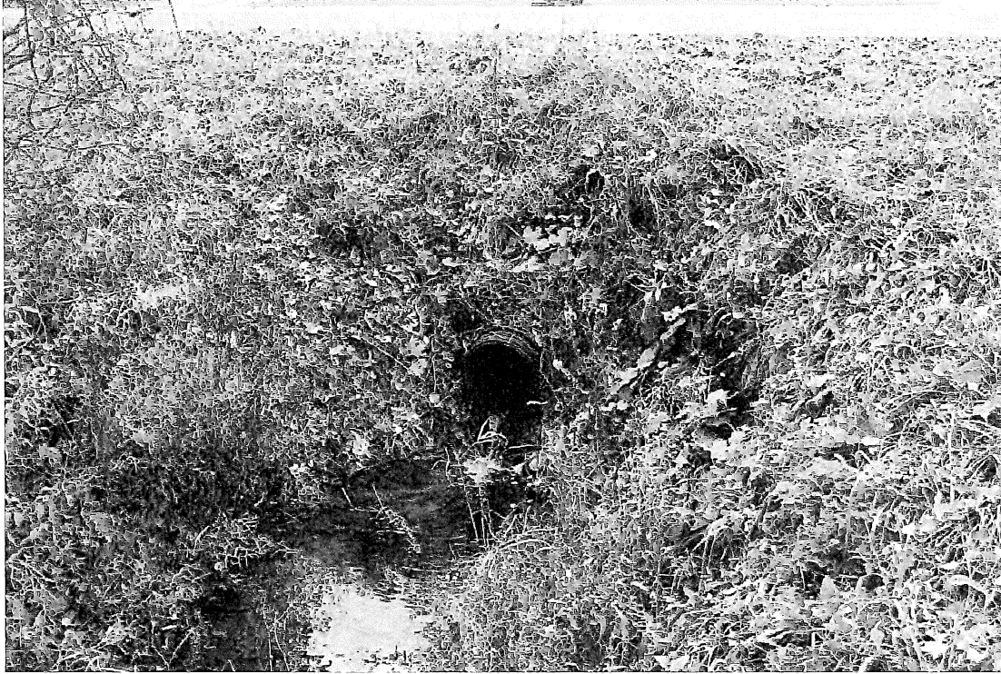
Picture #1 - Exit culvert from the end of the ditch catch basin; undersized; facing west
