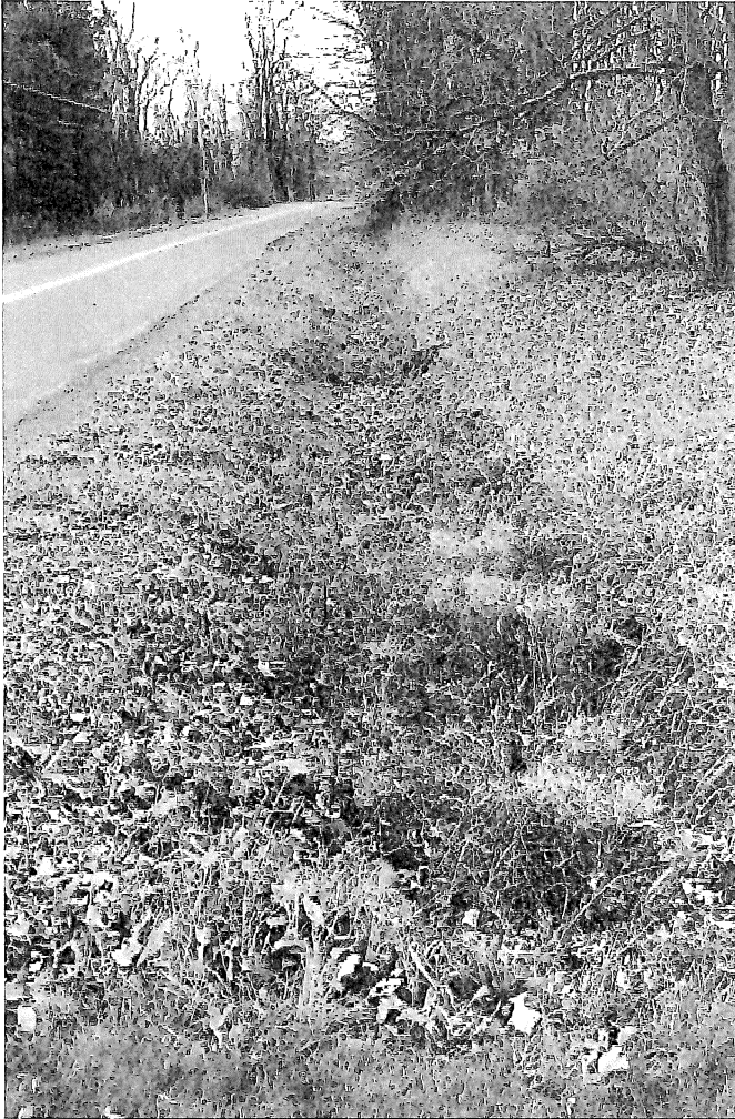
Picture #6 - Undersized, over vegetated ditching; facing south
