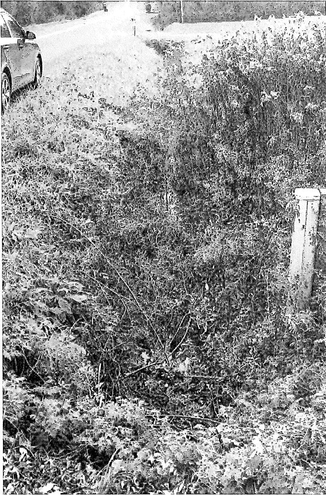
Picture #3 - Undersized, over vegetated ditching; facing south
