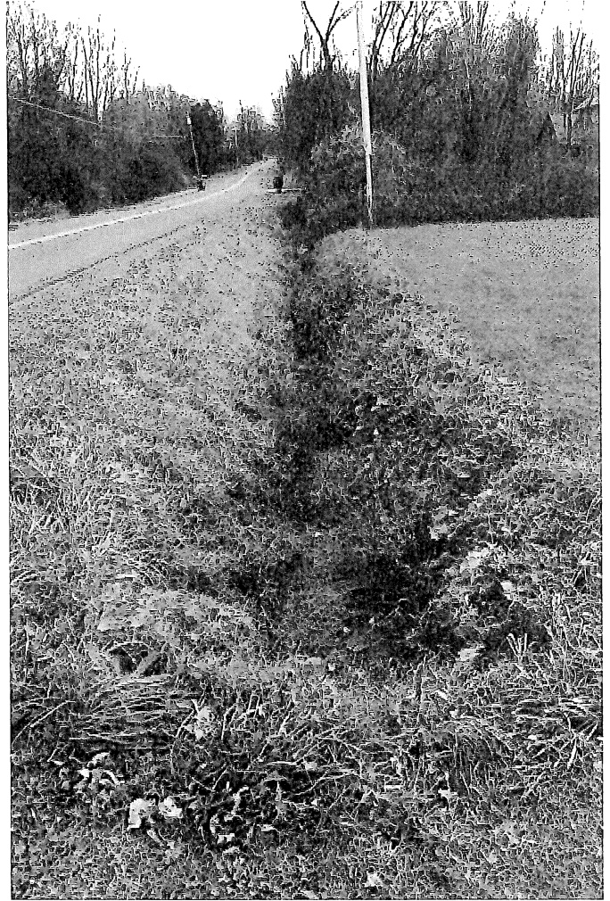
Picture #4 - Undersized, over vegetated ditching; facing south
