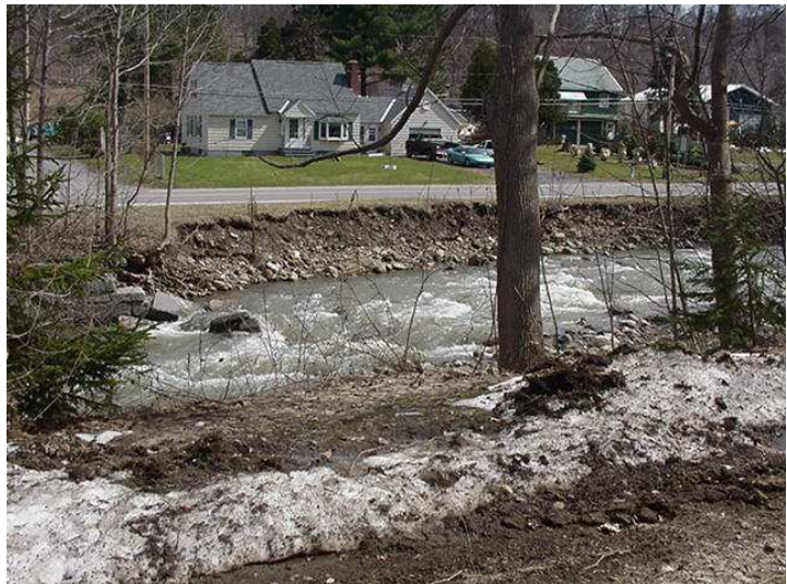
Figure 2: Collapsed Retaining Wall.
