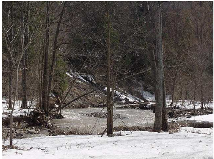
Figure 20: Bank slump near Fox residence.
