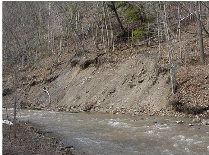
Figure 17: Typical stream bank erosion on Moyer Creek.
