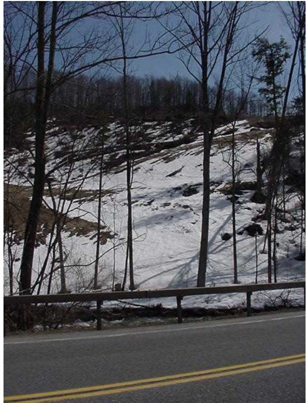
Figure 14: Potential area of runoff and sedimentation.
