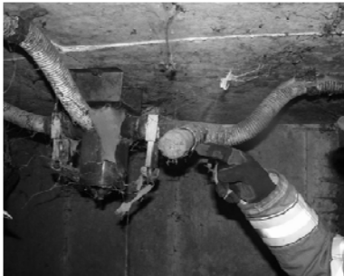
Gas injection port
