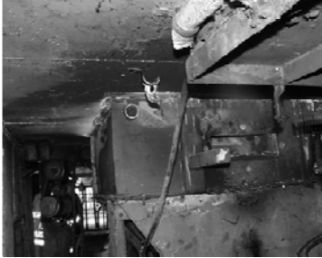
Notice melted breather pipes
