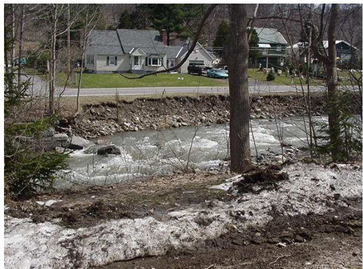
Figure 2: Collapsed Retaining Wall.
