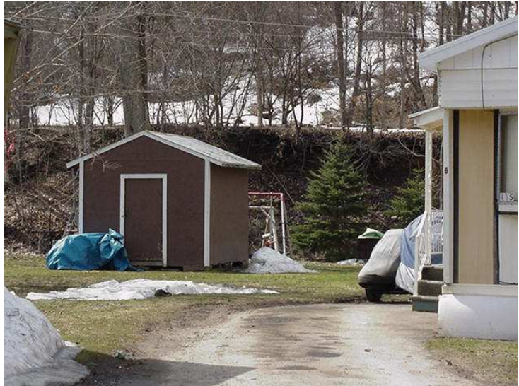
Figure 6: Severe bank cut on the western bank of Fulmer Creek.
