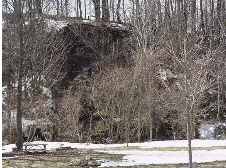
Figure 12: Stream bank erosion near McCready Road
