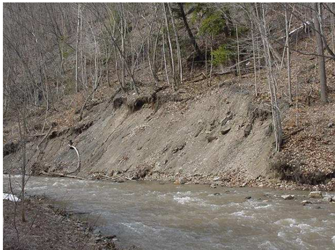
Figure 17: Typical stream bank erosion on Moyer Creek.
