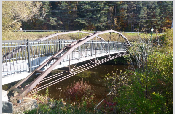
An original bowstring cast-iron truss bridge carries the trail over the canal just south of Main Street in Boonville.
