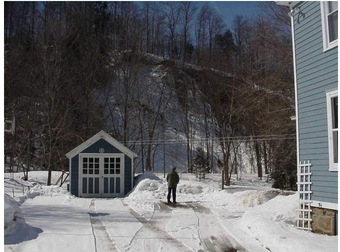
Figure 3: Severe bank slump behind the Bielanski residence.
