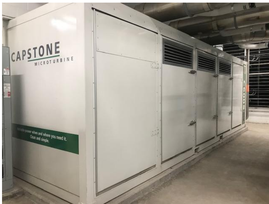
Figure 2. New Capstone microturbines at the Oneida County Water Pollution Control Plant. Source: Oneida County.
