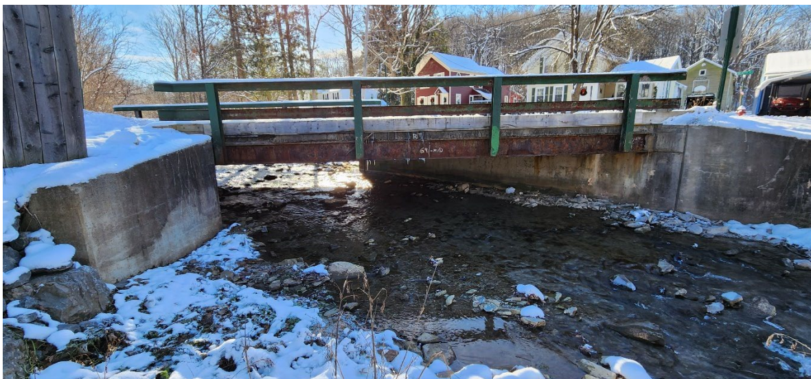
Figure 7-14. Downstream view of the Beatty Avenue bridge in the Sherman Brook corridor.
