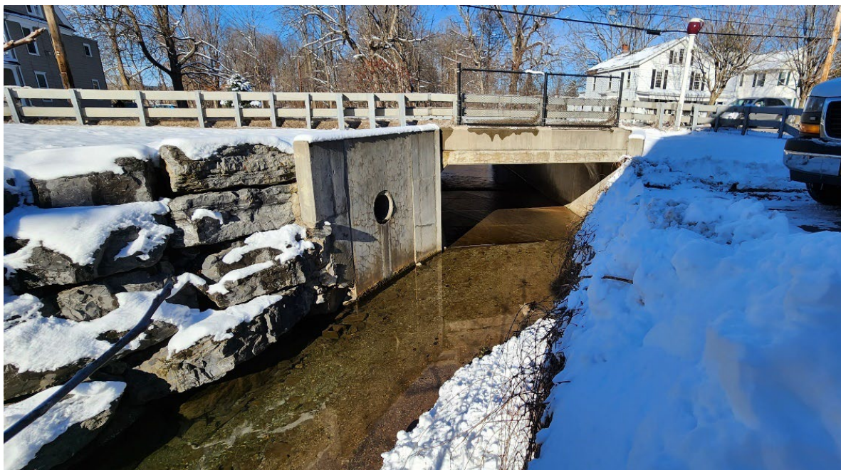
Figure 7-23. Upstream view of the Utica Street culvert in the Sherman Brook corridor.
