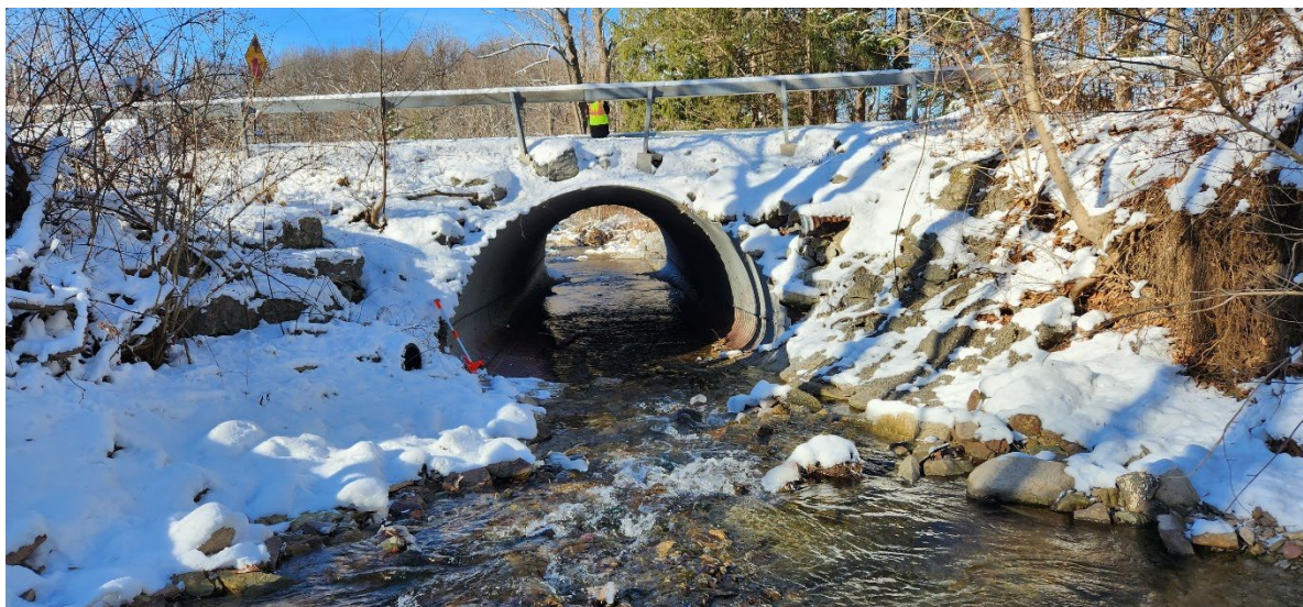
Figure 7-6. Upstream view of the New Street Culvert in the Sherman Brook corridor.
