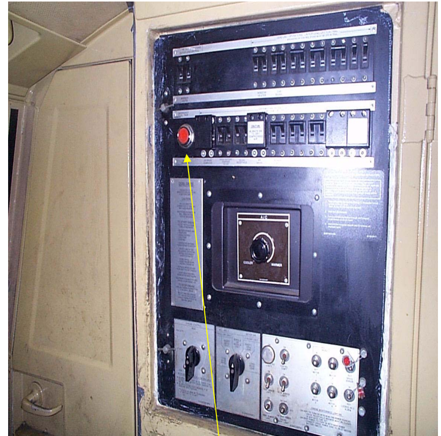
Emergency fuel Trip (shut off) on the panel on the rear wall of the engineers compartment
